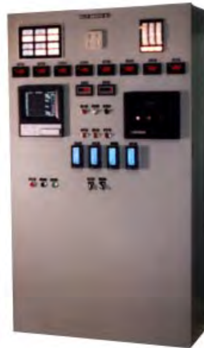
Above: TYPICAL PROCESS INSTRUMENTATION PANEL
